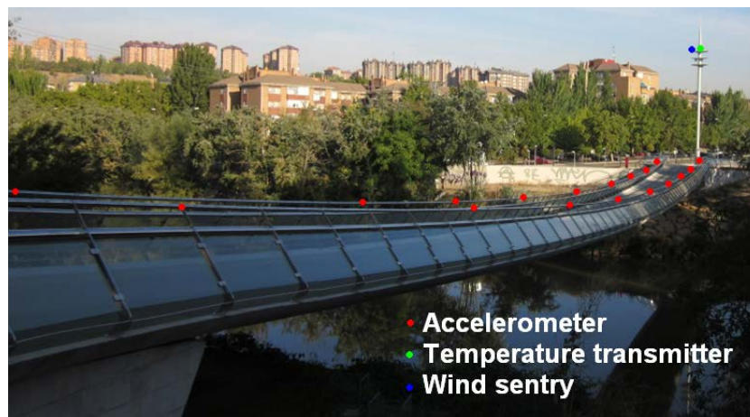
Figure 2. Monitoring system. Distribution of sensors.
